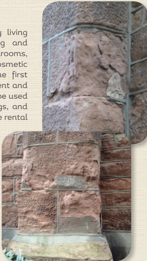
Examples of degraded stonework.
